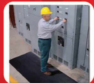
Electrical Mat (As per IS 15652)
