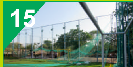
ELECTRICAL CABLING & FLOODLIGHTS
